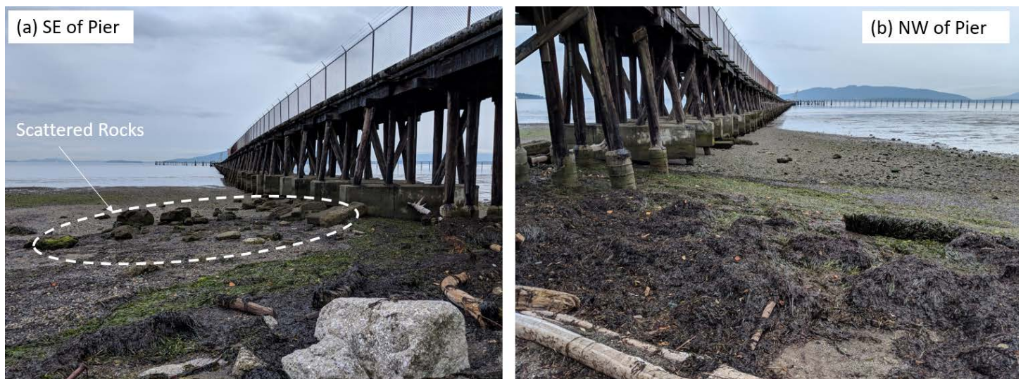
Figure 10: Ground photos on southeast (SE) and northwest (NW) sides of the pier from an October 5, 2018 site visit by a M&N coastal engineer.
